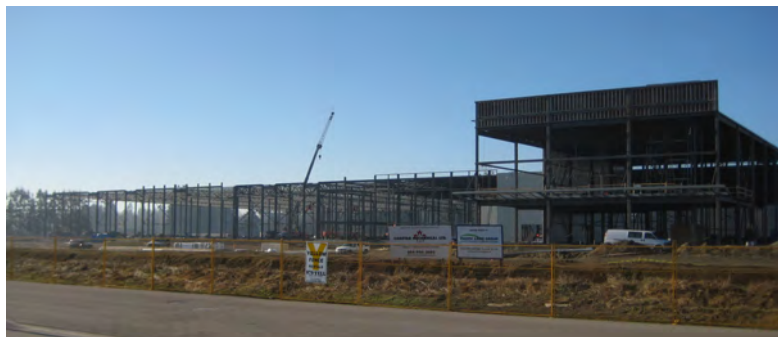
After completing one of the largest land transactions of 2008, Loblaw's has begun construction of their 421,000 sq.ft. fresh produce distribution facility in Campbell Heights, Surrey.
